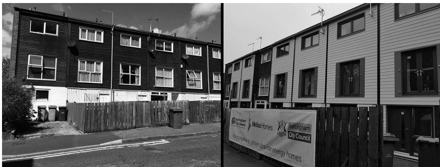
FIGURE 7.1 The ‘2050 homes’ in Sneinton, Nottingham, before (left) and after (right) retrofitting. The houses were renovated to reduce energy loss. REMOURBAN funding allowed Nottingham City Council to secure a higher energy efficiency standard than originally planned.
