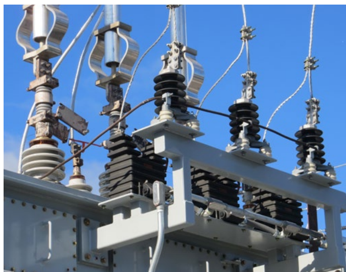
Silicon Valley Power. Source: American Public Power Association on Unsplash
